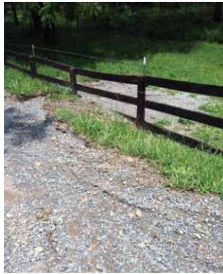
Left: Road conditions on Poor House Road after flooding.
