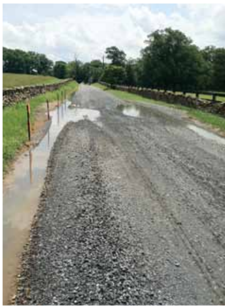
Above: Standing water on Millville Road near Unison after heavy rains shows the need for greater attention to maintaining and preserving our rural roads.
